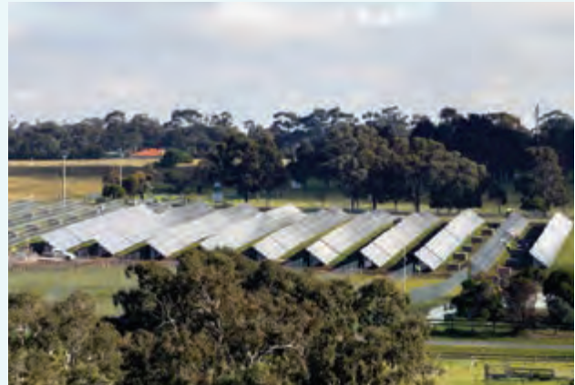
Solar array development, Melbourne Airport, Australia
