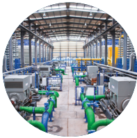
Utilities: Water, Heating & Telco
